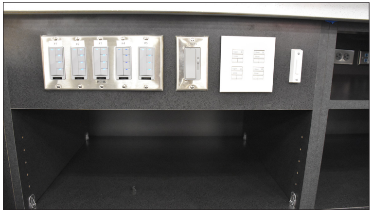
Central lighting controls, shade controls and bell to call for help at service desk
