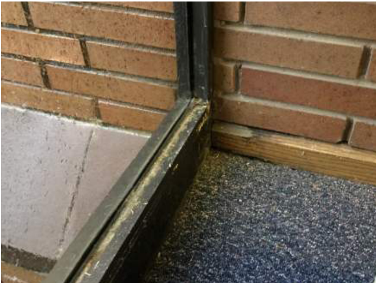
Water damage seen in window sill, wood base and carpet discovered during an FCA at a public library
